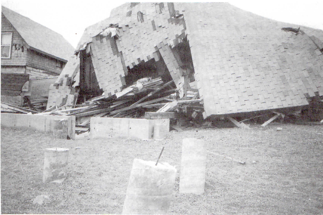
Figure 27. A house moved off its foundation in Scituate, Massachusetts. Photo courtesy of Pat Viets.
